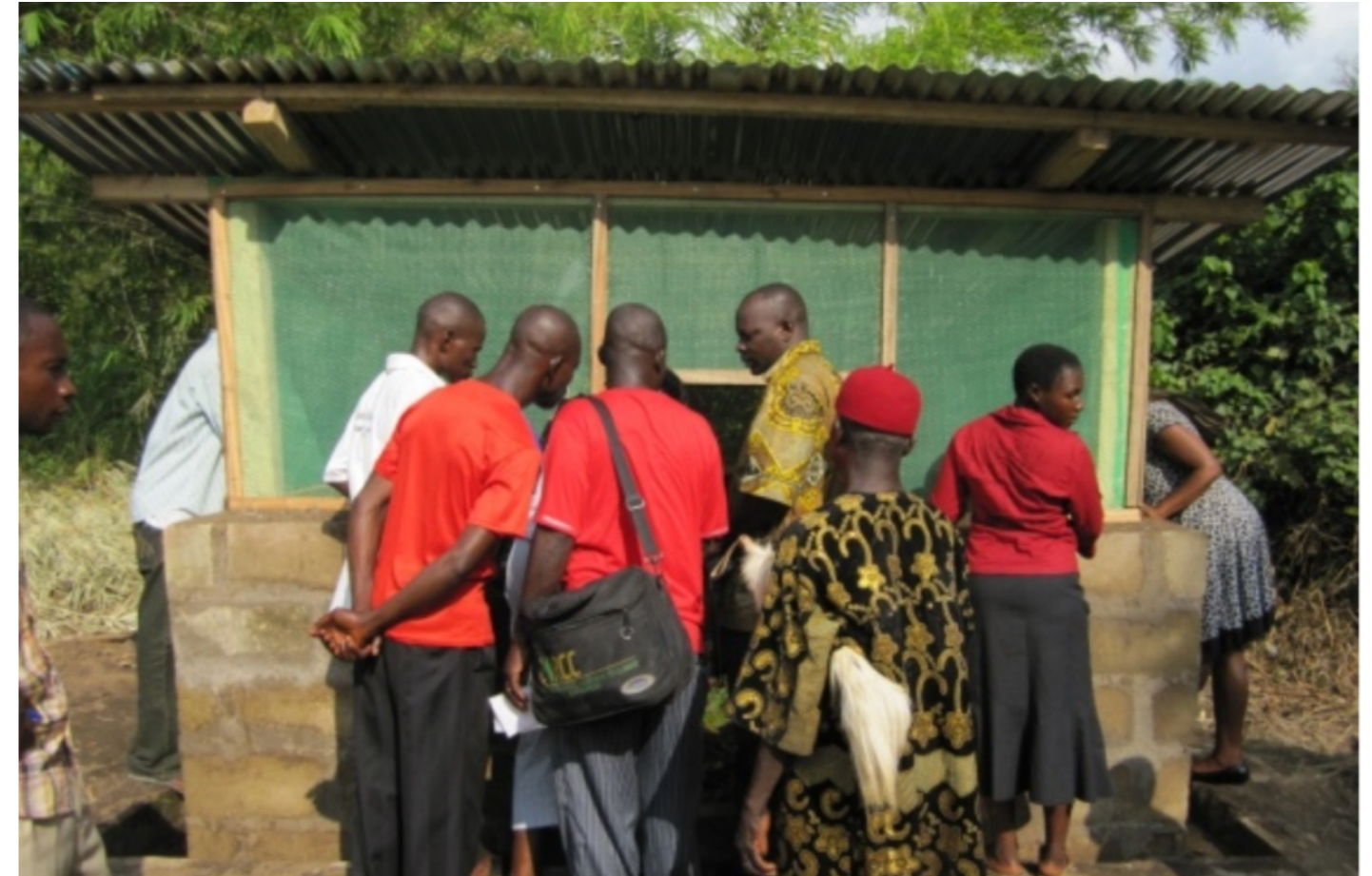
Structure built by the community to house farmed snails in Bebi IV
