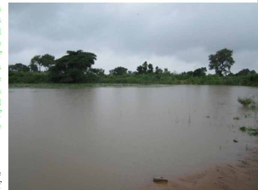
Rehabilitated dam in Daudu to provide water for washing, irrigation and drinking
